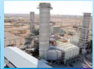
AMAL Heat Recovery Steam Generator (HRSG) project for PDO
